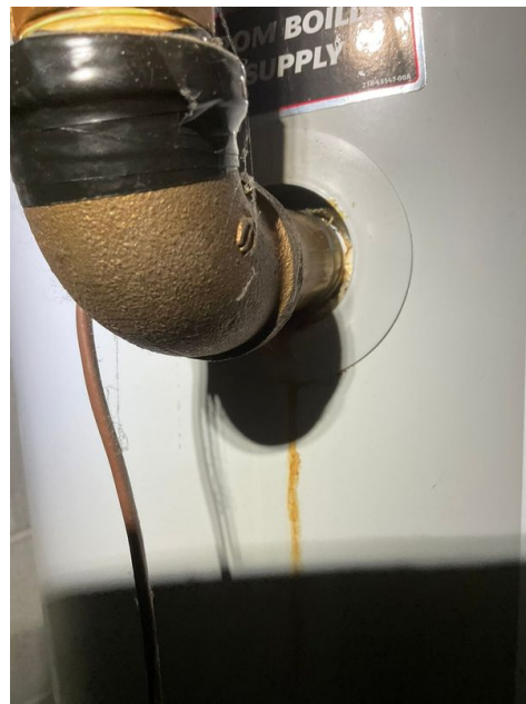
And weeping/corrosion at boiler inlet
