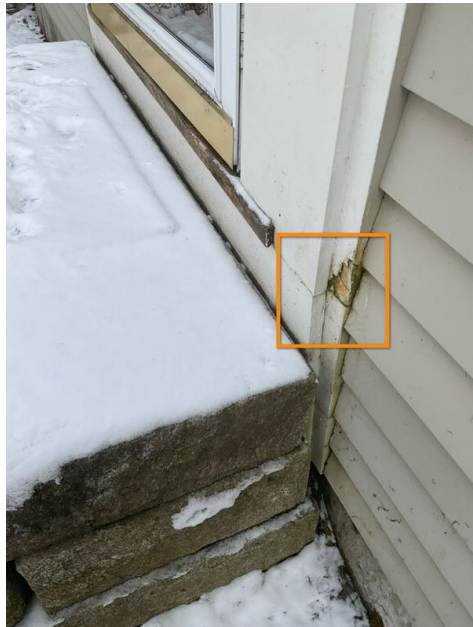
Decay at front entry
