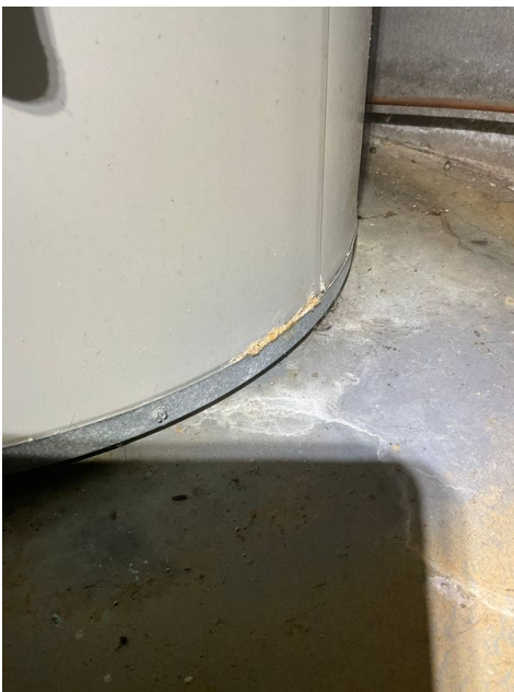
BW tank with base corrosion
