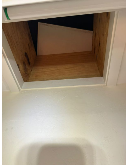
Bare hatch is the weak-point in attic insulation
