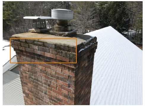
Early moisture absorption at mortar joints
