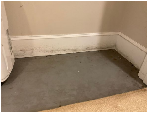
Light staining at basement closet
