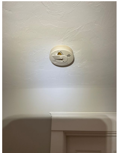
Expired and disconnected in second hall
