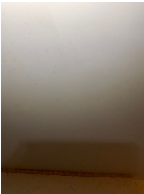
Light staining on ceilings (hard to see in picture)
