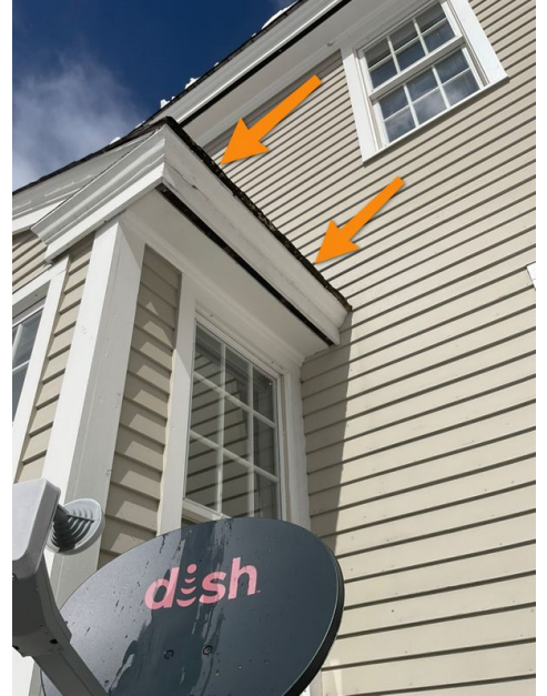
Uncapped cedar absorbing a lot of moisture
